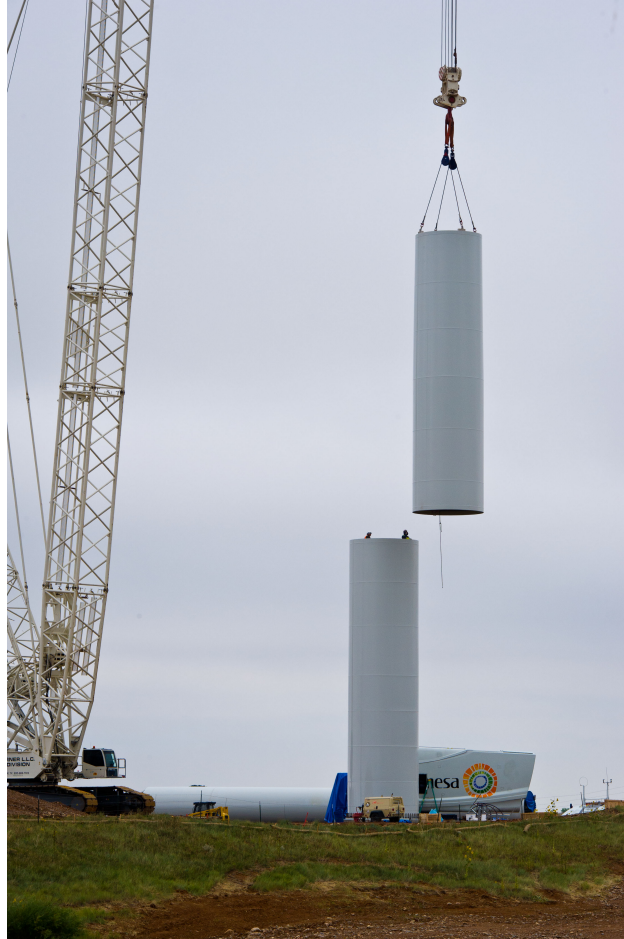
Figure 2.10: On-site assembly of steel wind turbine tower sections. Photo by Dennis Schroeder, NREL 20843.
