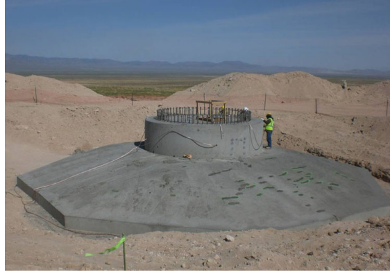
Figure 2.9: A typical onshore wind turbine foundation, before backfilling. Photo from the Bureau of Land Management, US Department of the Interior.
