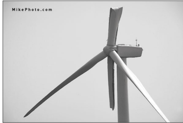
Figure 2.2: Structural failure in a wind turbine blade. Photo by Mike Lascut, used with permission.
